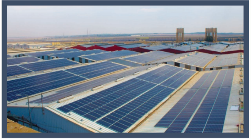
Gaza Industrial Estate (GIE) Produces 7.3 MW
